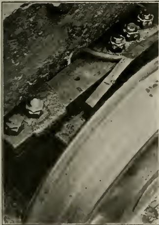
LOCOMOTIVE TRUCK, LEFT SIDE BROKEN AND WELDED WITH U S L ARC WELDER WITHOUT REMOVING
